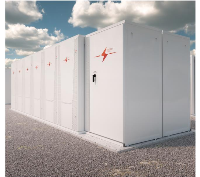
Energy Storage Systems
